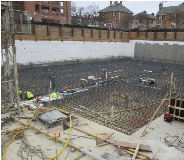
Photo 4. Example of pre-applied TPO system waterproofing in a “Bath tub” design.
