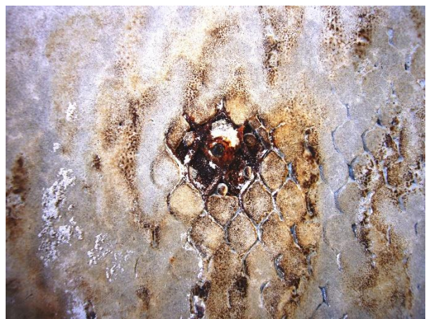
Corroded and failed lath fastener
