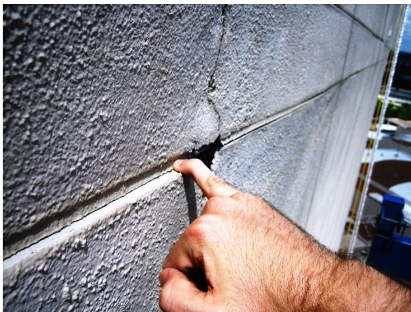
Stucco displaced due to failed lath fasteners
