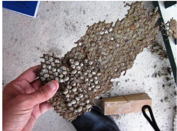
Severe corrosion of lath found at large unsealed crack in stucco
