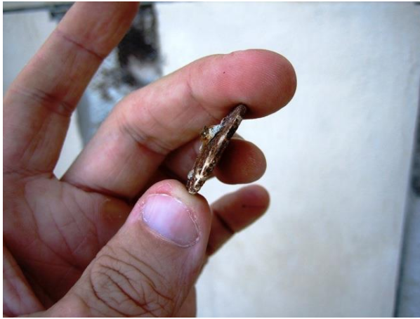
Failed lath fastener
