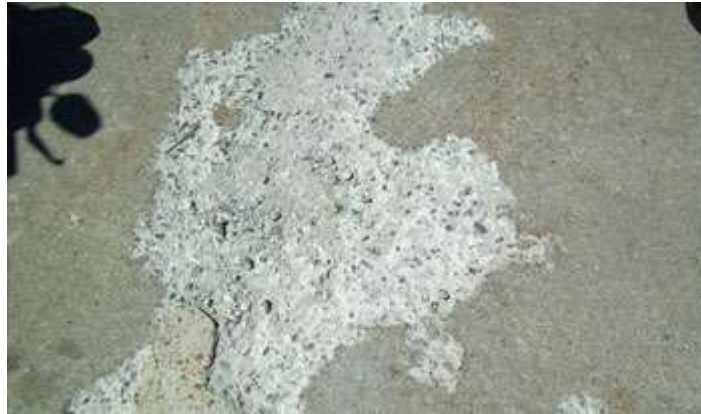
Photo 4. Example of Concrete Surface Scaling
