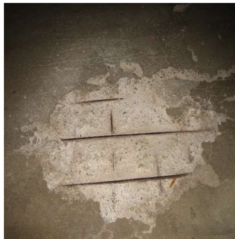
Photo 1. Typical corrosion induced spall at a reinforced concrete slab due to chloride infiltration.
