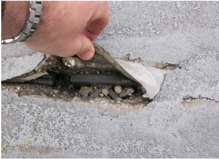
FAILED SEALANT JOINT EXPOSING A SHEAR CONNECTION
