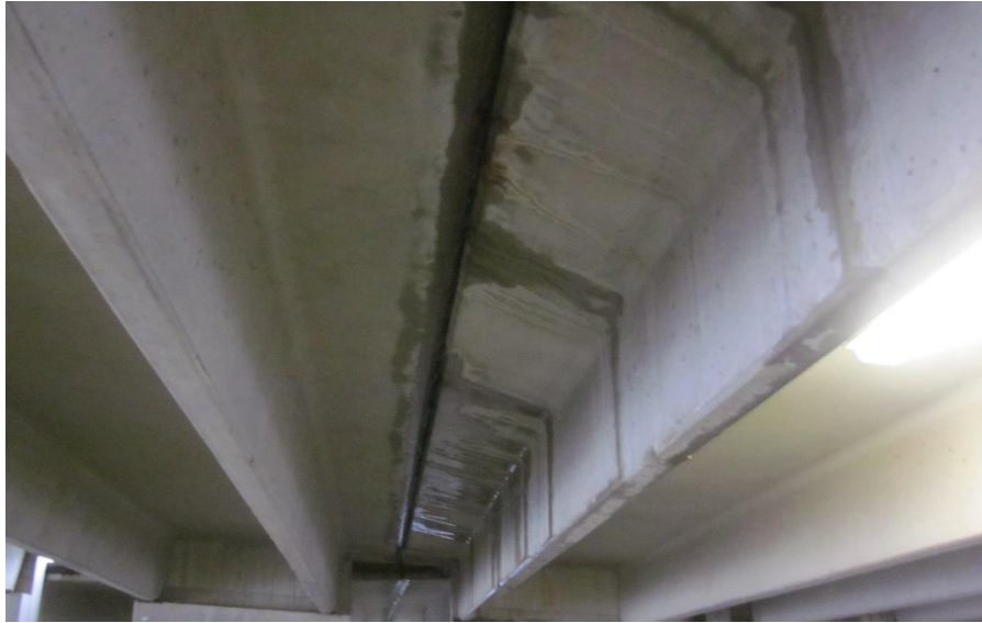
WATER LEAKAGE THROUGH FAILED SEALANT JOINT
