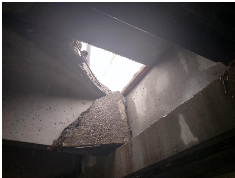
FAILED CONCRETE AT A DOUBLE-TEE FLANGE CORNER
