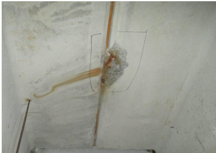
CORROSION RELATED SPALL AT SHEAR CONNECTION
