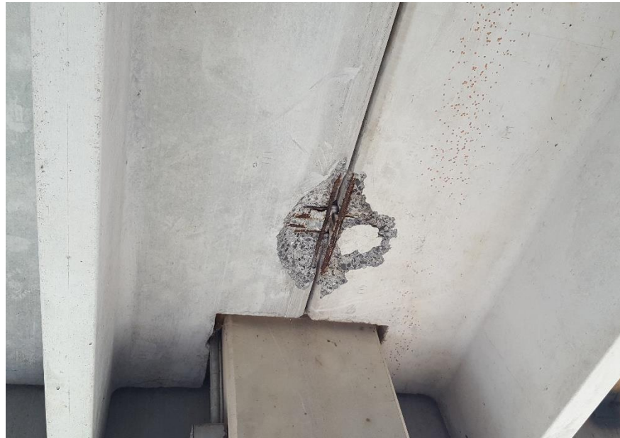
CORROSION RELATED SPALL AT A SHEAR CONNECTION
