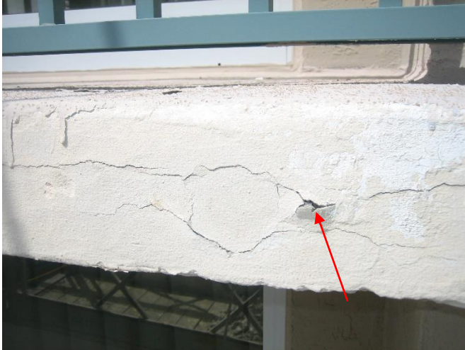
Photo 3 – Close view of a balcony slab edge with cracks and deteriorated coating. This condition permits water and oxygen to reach the embedded steel PT anchors and mild reinforcing steel.
