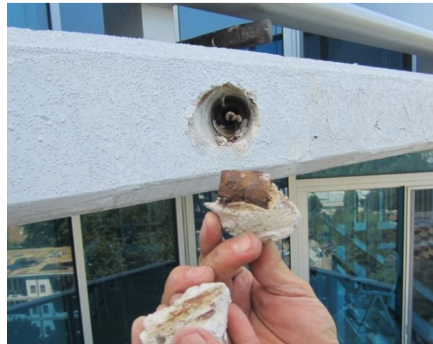
Photo 2 – removed grout revealing corroded wedges and anchor due to water intrusion at the grout pocket
