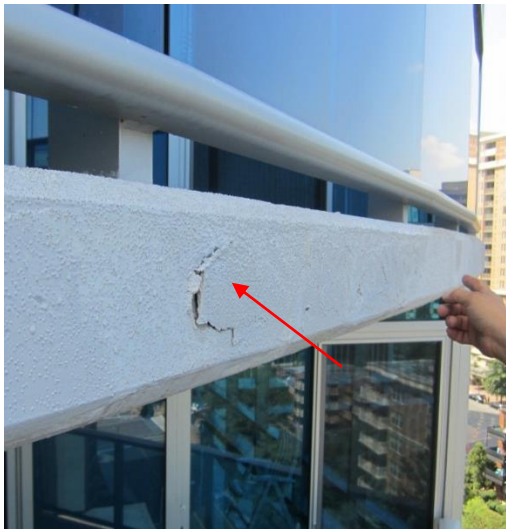
Photo 1 – debonded grout over anchor pocket
