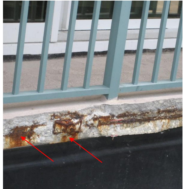
Photo 4 – Balcony slab edge after delaminated concrete was removed revealing corroded PT anchors and mild reinforcing steel.
