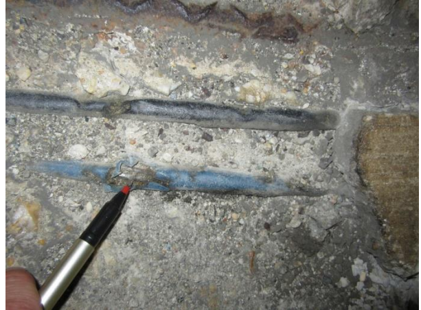
Photo 7 – A damaged PT tendon on a garage mat slab top surface. The previously delaminated concrete has exposed this cable to damage from vehicular traffic, water and deicing salts.
