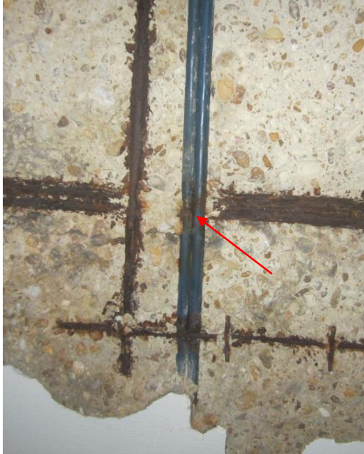
Photo 6 – View of garage slab bottom surface after delaminated concrete had dislodged and fallen from the soffit revealing corroded PT tendons and mild reinforcing steel.
