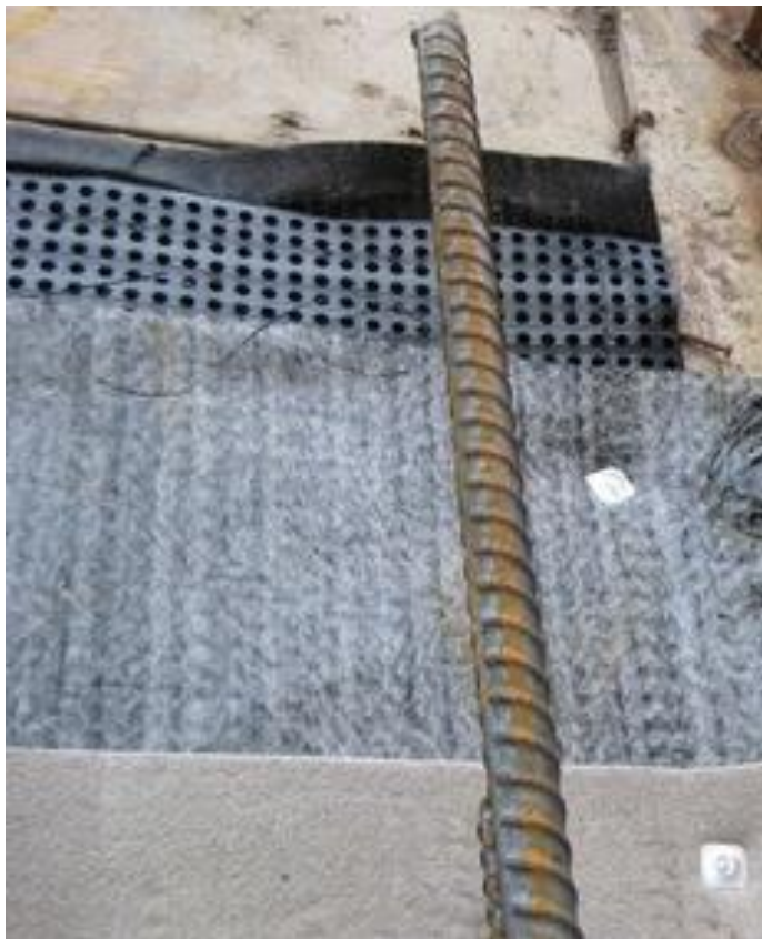
Photo 2. Close view of Bentonite System
